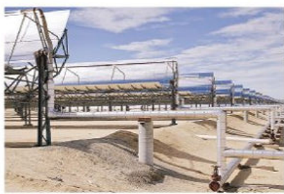
ENERGY: Solar collectors harness energy to generate electricity in Harper Lake, California. US venture capitalists are especially interested in clean energy.
